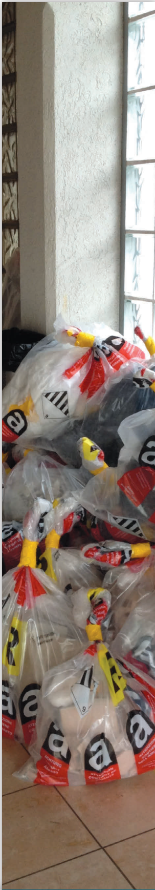
Asbestos bagged and labelled.
