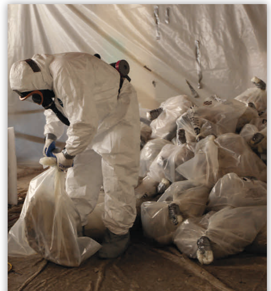
Asbestos bagged twice.
